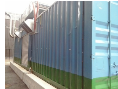
Outside of Unit
